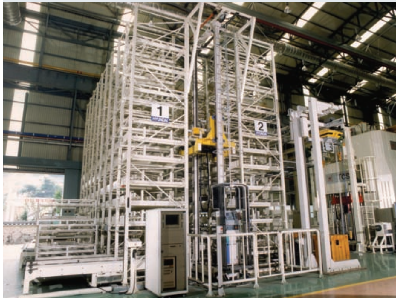
● Unit Rack AS/RS
