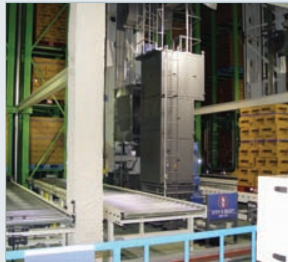
● Stacker Crane (50mH)
