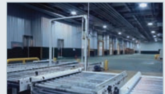
● Conveyor- I for In & Out
