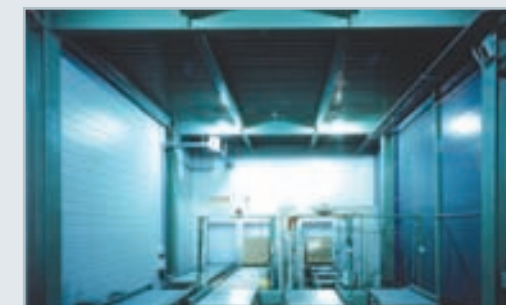
● Conveyor- II for In & Out
